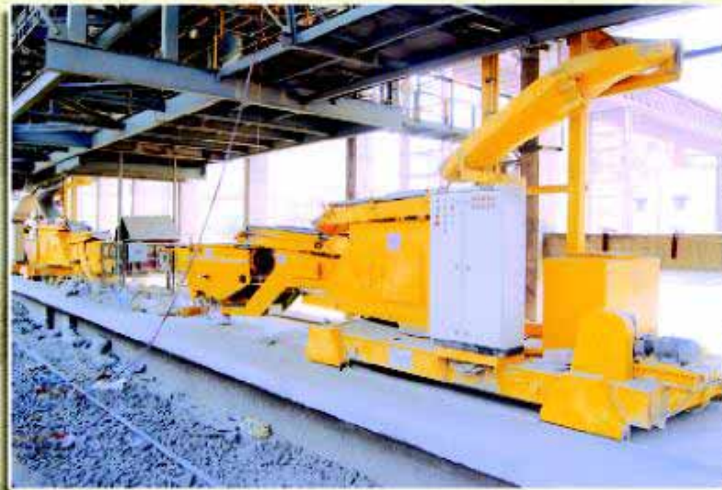
The newly installed wagon-loading machine at Durgapur, in addition to the existing infrastructure
