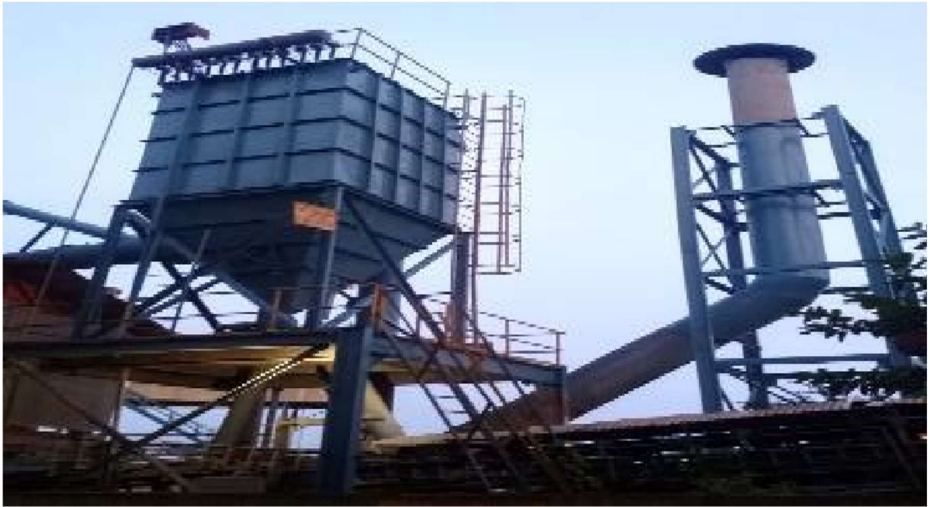
Bag Filter installed at transfer points
