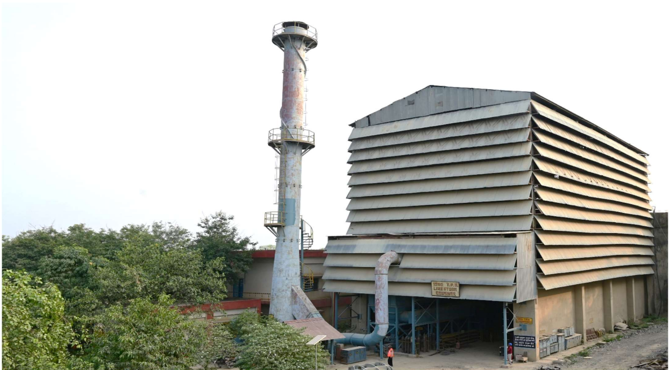
Bag House installed at covered Crusher
