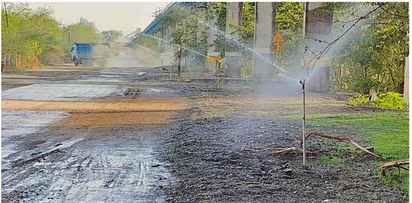
Fixed Water Sprinklers along Haul road
