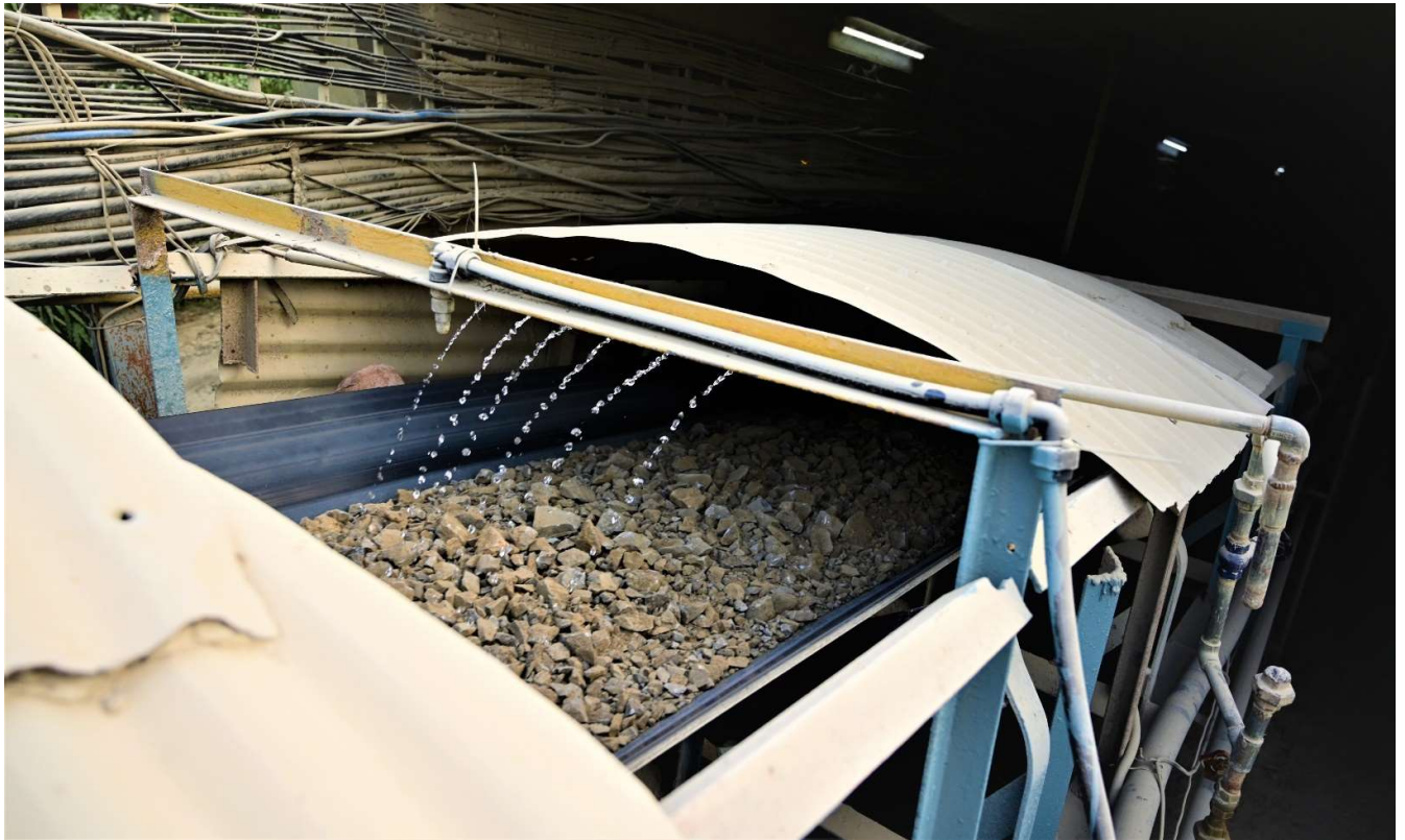
Water spray system installed at conveyor belt
