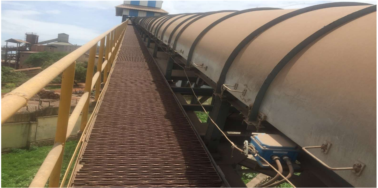
View of Covered Conveyor Belt
